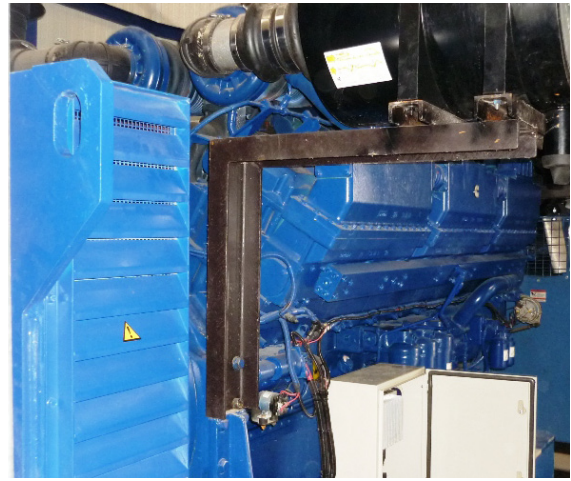
A generator set powered by a Cummins G-Drive QSK78-G8 engine provides emergency backup for the pumps
