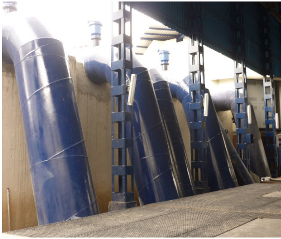
The re-equipped plant has double the capacity to pump water
