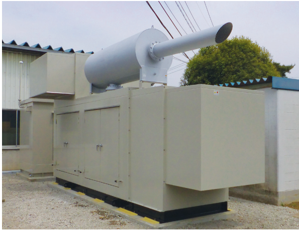
TDS supplies containerized units for mission critical sites
